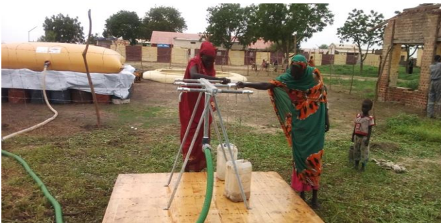
Newly installed SWAT system in Renk, Upper Nile. ©World Vision/August 2017
