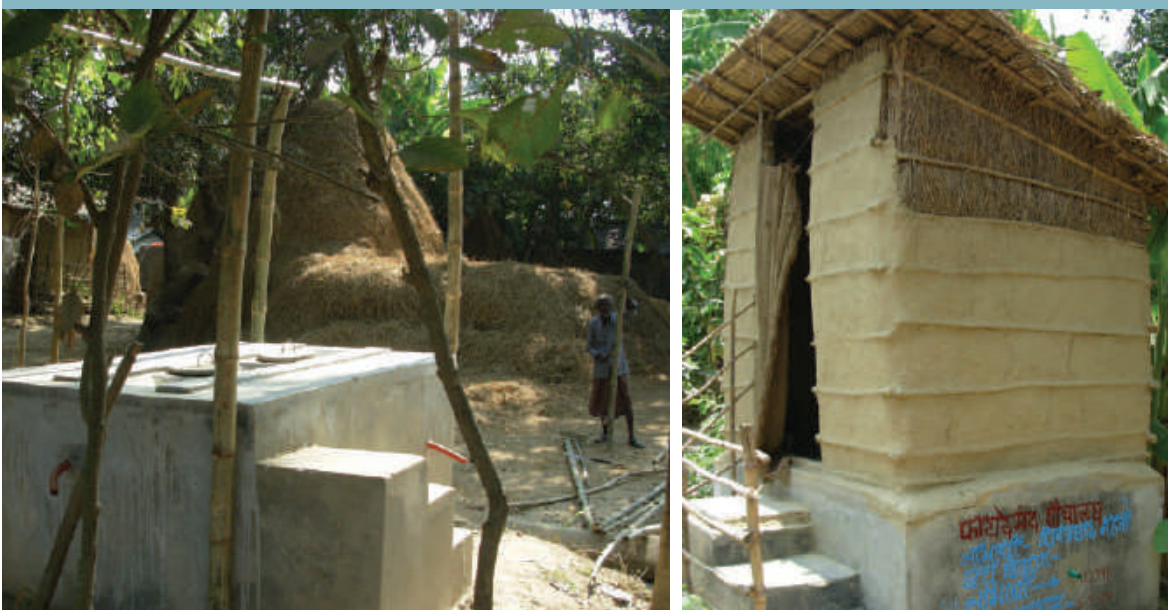
This project in Bihar, India, tackled the financing issue by providing the concrete substructure for flood-resistant toilets, while households were responsible for building the superstructure. Photo: Kim Andersson
