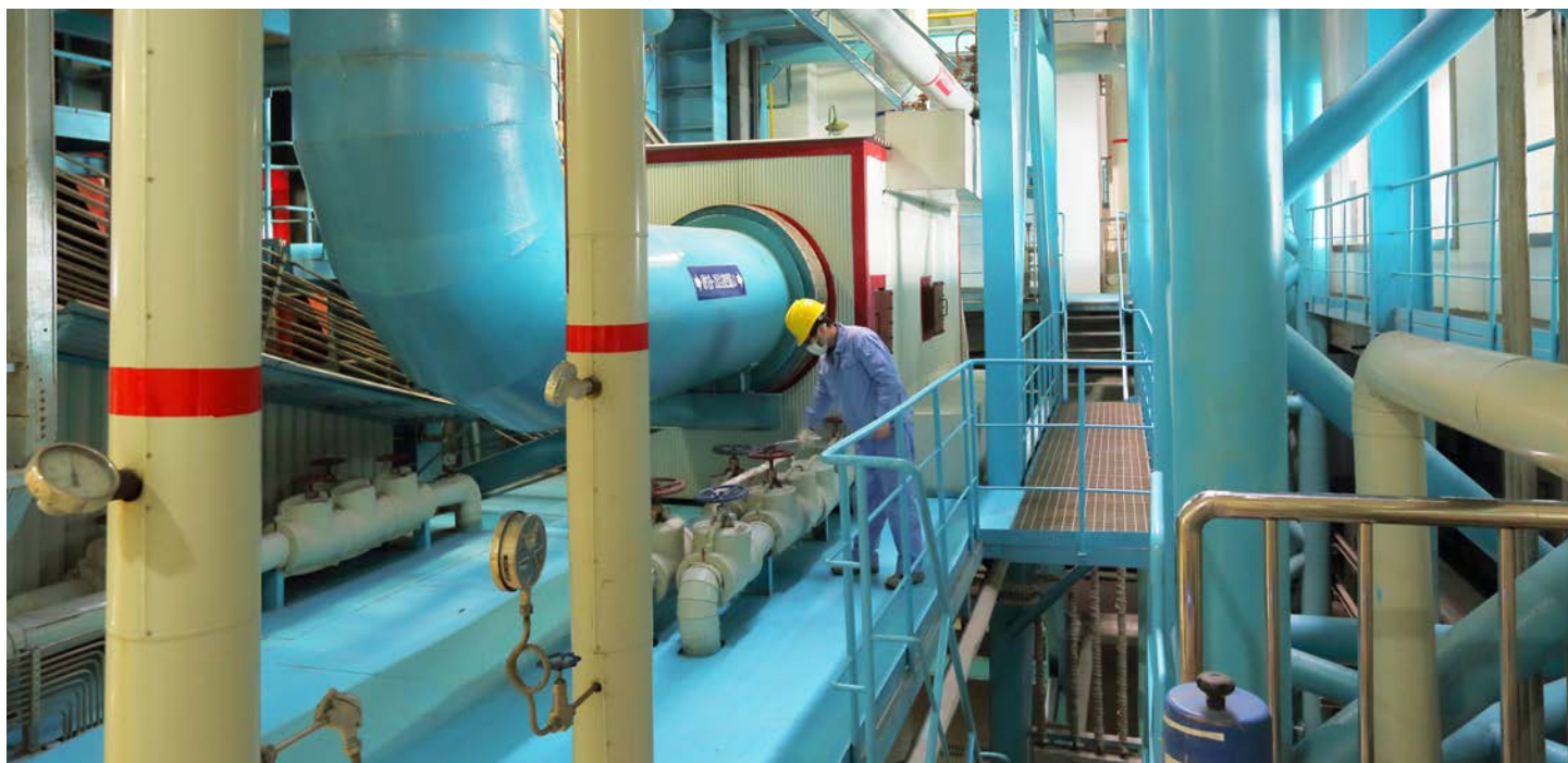
This ADB-supported waste-to-energy plant in Suzhou in the PRC has helped create better living conditions in the city. In 2020, the bank committed $206.6 million to support waste-to-energy and other environmental initiatives in Hebei province.
