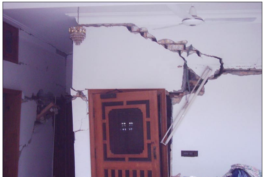
Figure 7. Severely damaged unreinforced brick masonry wall in Muzaffarabad.
