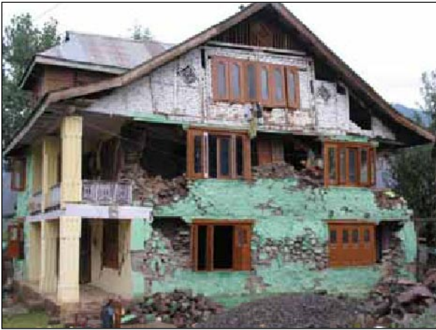
Figure 12. Timber-laced masonry in gable wall suffered little damage, whereas extensive damage in stone masonry wall rendered the building unsafe at Uri.
