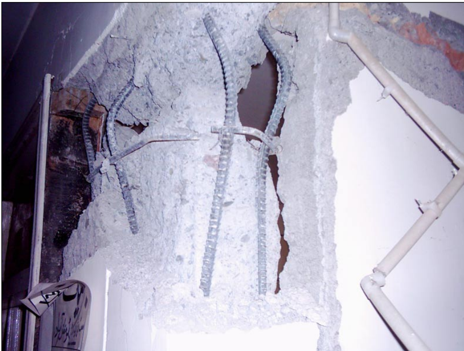
Figure 9. Formation of plastic hinge in the column near the beam-column joint in a hospital building in Mansehra.
