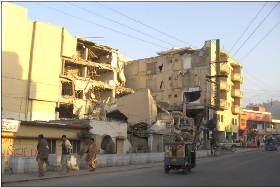
Figure 8. Collapse of Sangam Hotel, an 5 storeyed RC framed building in Domel, Muzaffarabad (Latitude N34° 21.3' Longitude E73° 28.3').
