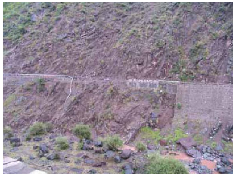
Figure 13. Landslide on NH1A near Uri disrupted the road traffic.
