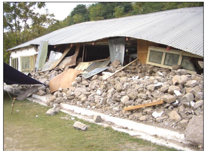
Figure 5b. Collapsed stone masonry building (metal roof)
