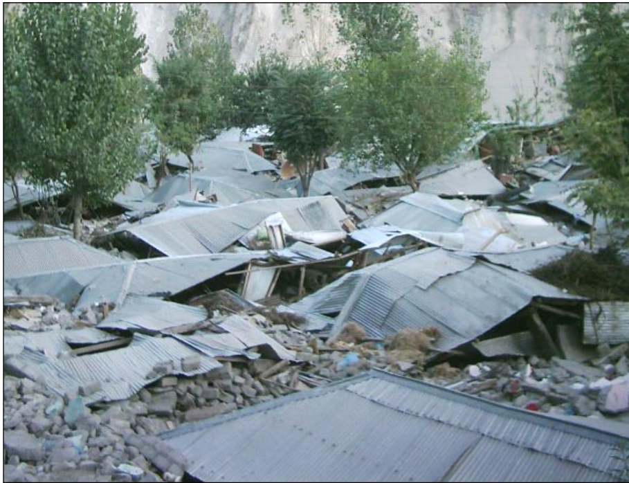
Figure 6. Collapse of unreinforced concrete block masonry houses in Kamsar near Muzaffarabad (Latitude N34° 24.6' and Longitude E73° 28.5').
