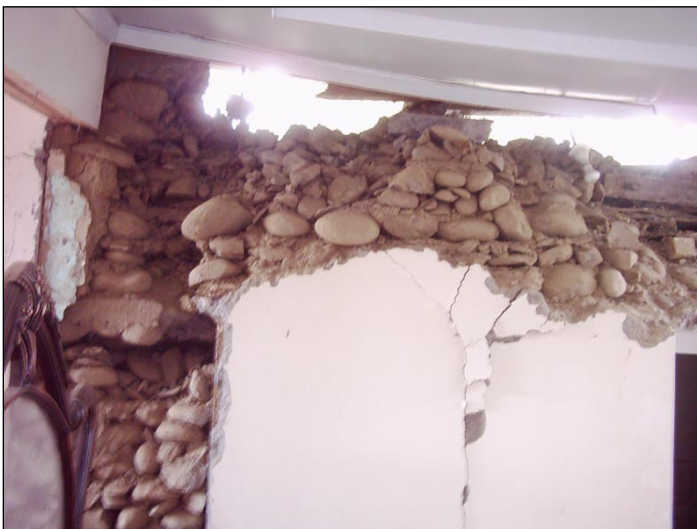
Figure 5a. Failure of unreinforced stone masonry walls in Muzaffarabad.
