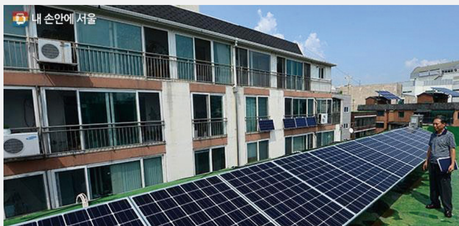
Figure 44 Mini solar panels installed in Sibjaseong Energy Self-Sufficiency Village (Source: Seoul Metropolitan Government, 2017)
