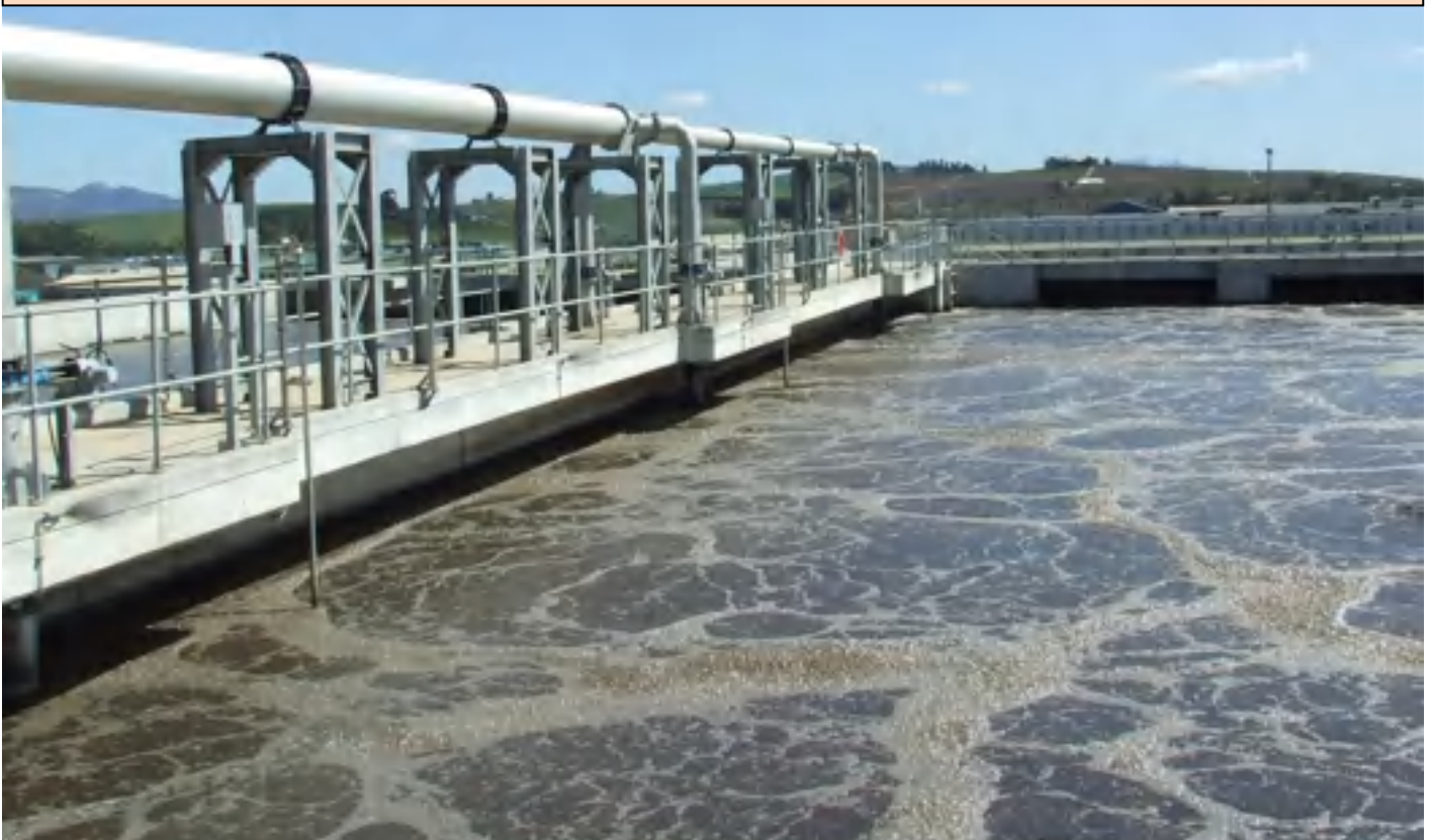
Drakenstein continues to impress. The Wellington WWTW aeration and works in general affirm how a plant should be operated. The evenness of the aeration draws the Regulator to this picture – well done with your Green Drop Excellence.
