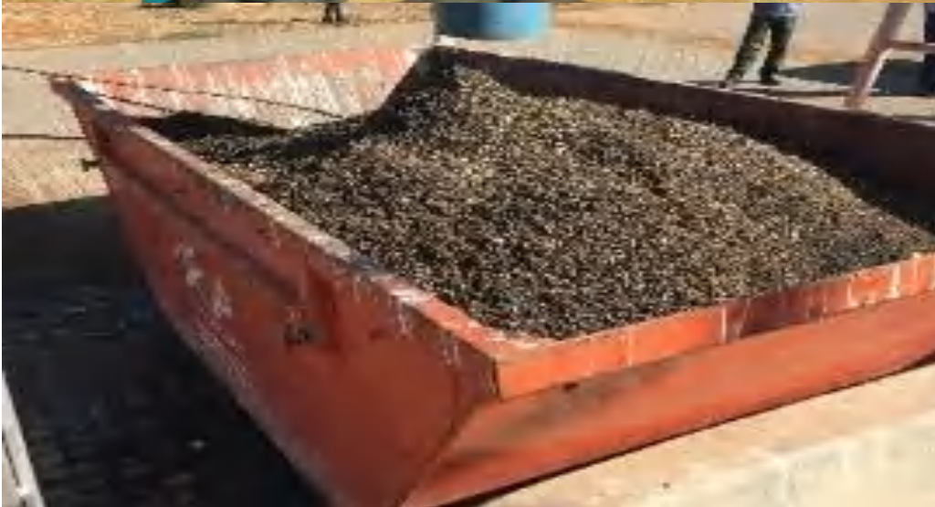
Despite considerable challenges facing the Rustenburg Municipality, the Boiketong WWTW attained a 100% score for degritting and removal to the Holfontein landfill facility. Well done to the general workers who make this happen.
