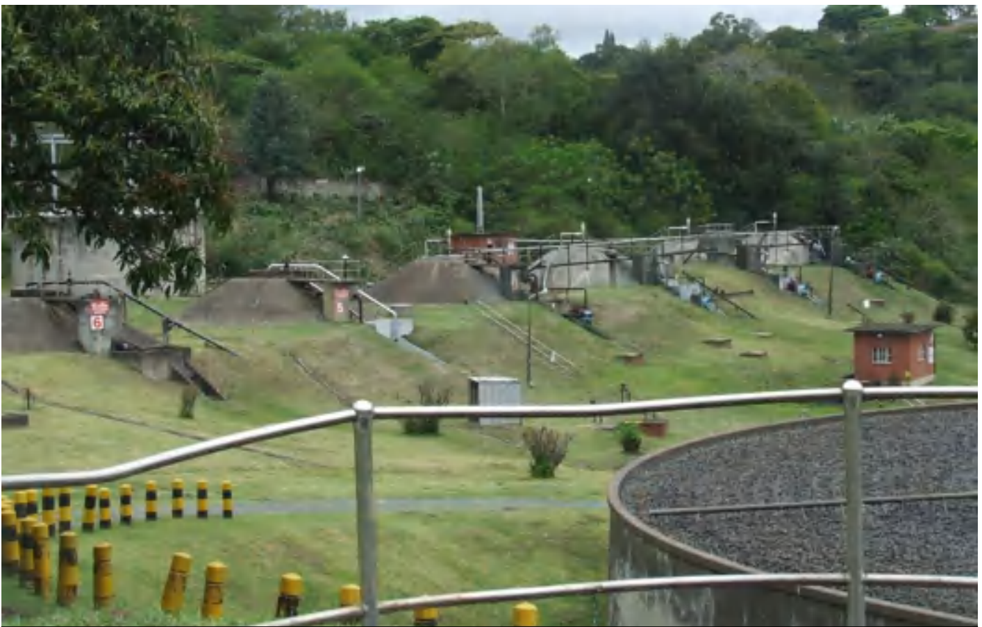
eThekweni Metro, Umbilo WWTW. The pristine nature of the works and infrastructure blends in with the conservation area, which the municipality ensure on a daily basis – 91% TSA score. Well done to this City.
