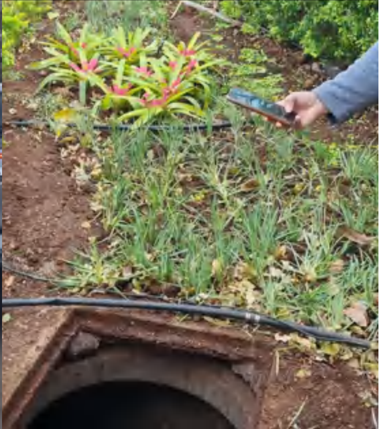
Excellent condition of sewer manholes and pipe condition, <45 minutes response time – well done to the Nkomazi team.
