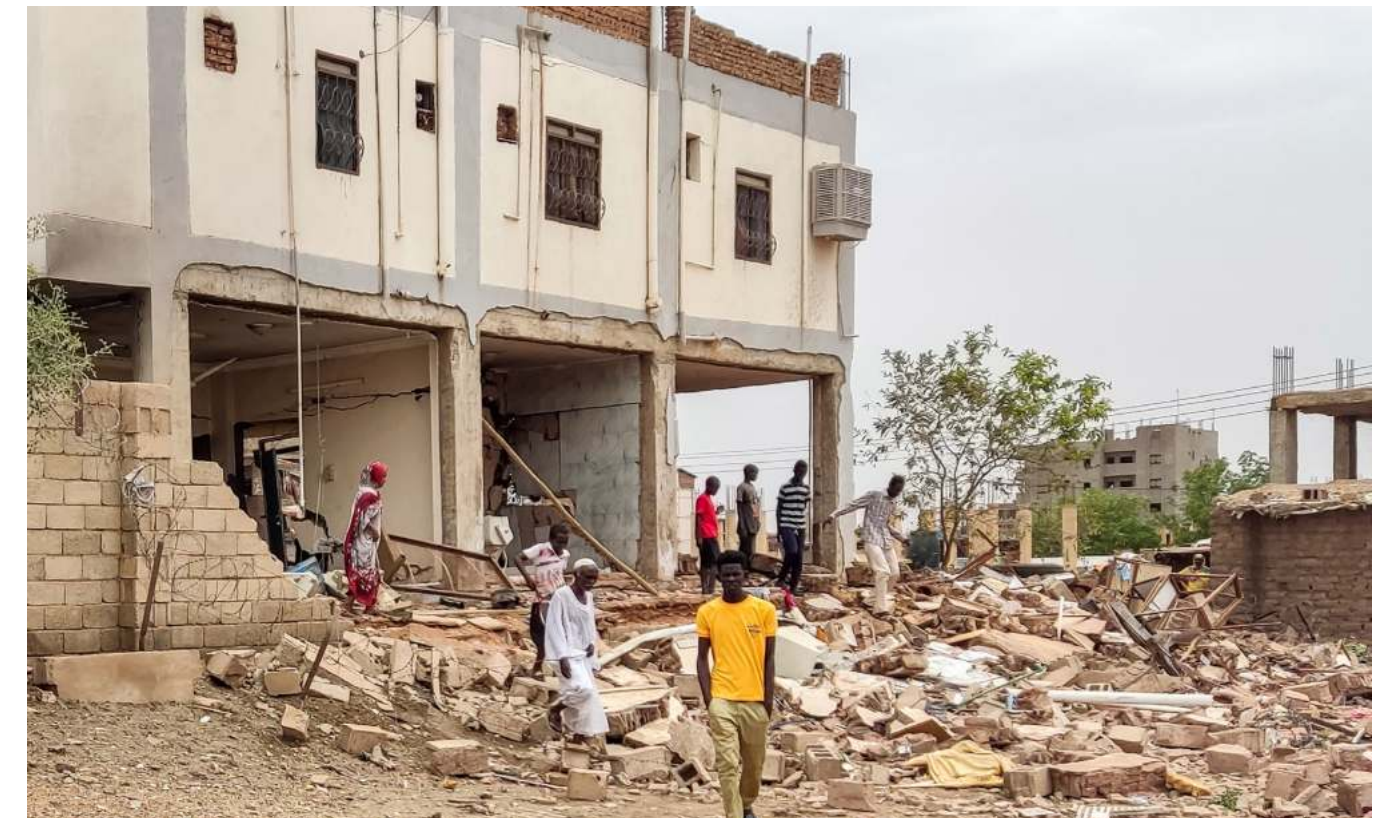
Men and women inspect the damage to a residential building in the Azhari district of Khartoum.
